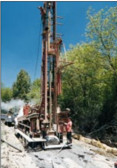
Drilling for the ground loop for Webster County High School's 500-ton GeoExchange system. It is the largest GeoExchange installation to date in West Virginia and the surrounding region.
